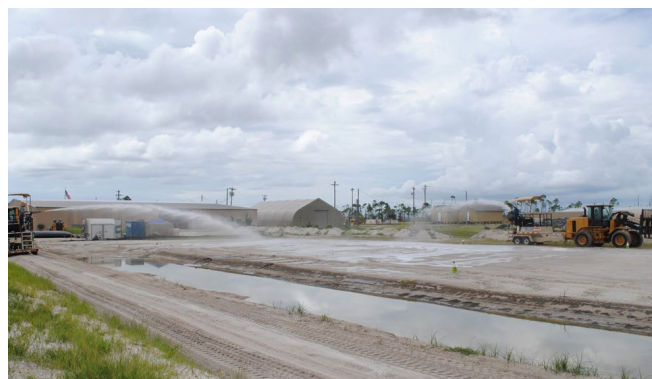
Biocement being sprayed on sandy soil at Tyndall, AFB. Photo Credit: Grace Bland
